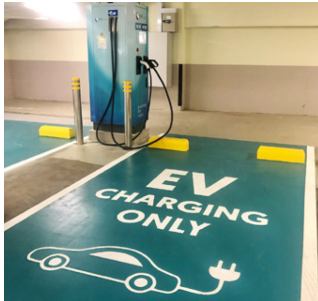
In partnership with SP Group, the direct current fast chargers at Republic Plaza can charge a car in 30 mins, bringing greater convenience to EV drivers in the CBD.
